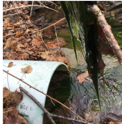
This outfall is partially submerged and a clean catch of its discharge is not possible. If tidal influences are strong, wait until low tide to sample. Additional options include: sampling upstream structures or using sand bags around the outfall to prevent contamination from backflow.
